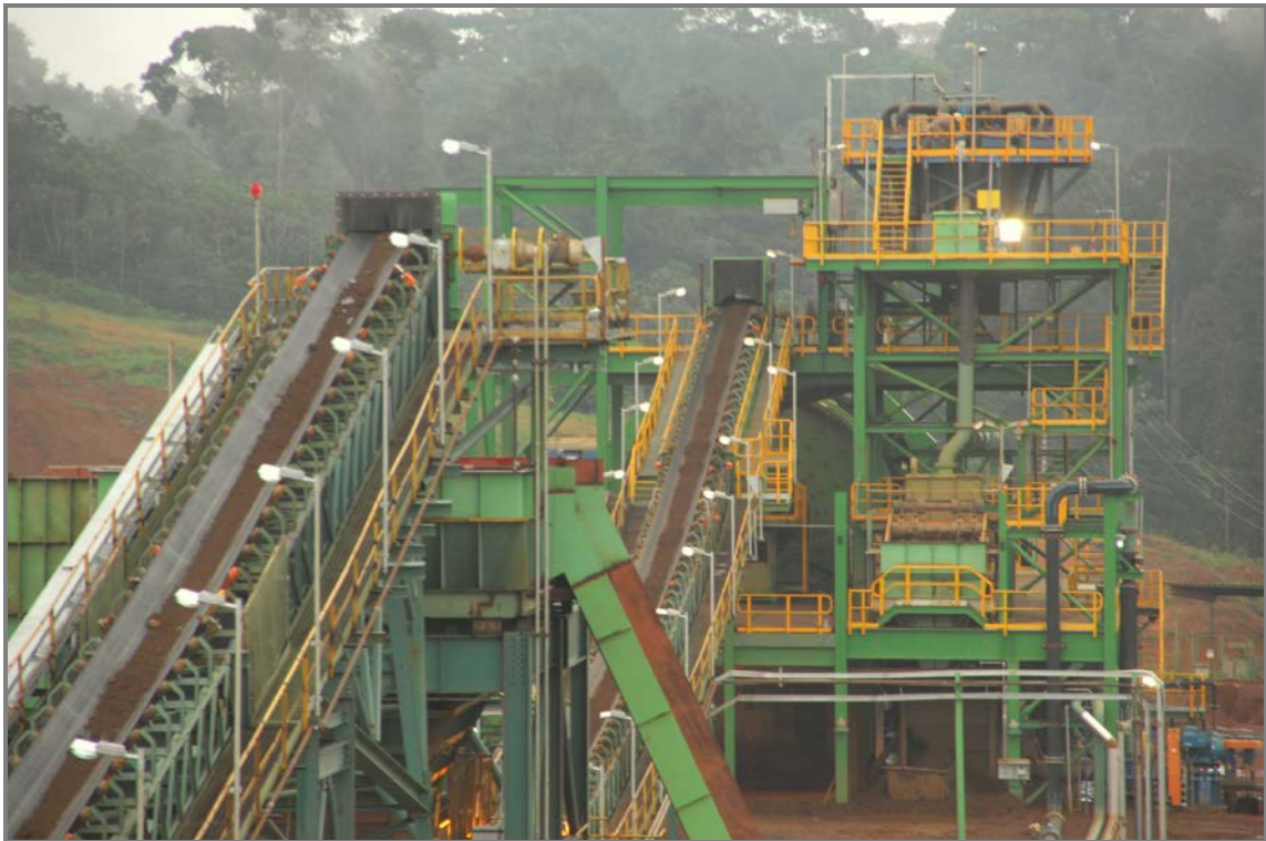
Photo 2. Crushing circuit in full operation
